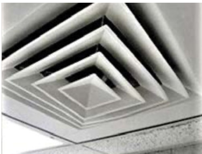
Figure 4. Typical supply air vent (diffuser).
